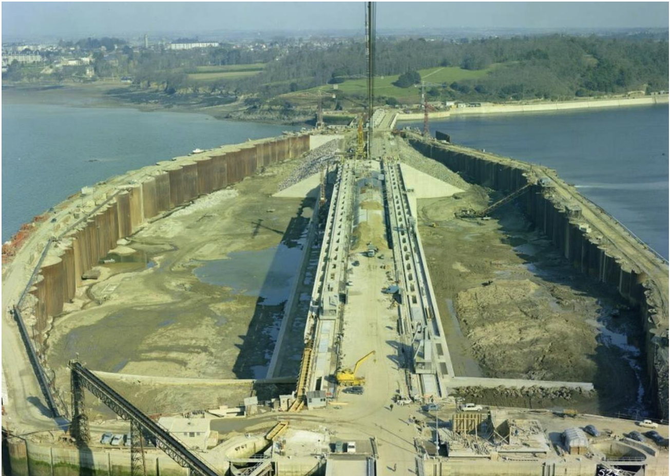
Plate 2.4: Example image of coffer dam La Rance Tidal Barrage under construction in a coffer dam (reproduced courtesy EDF)
